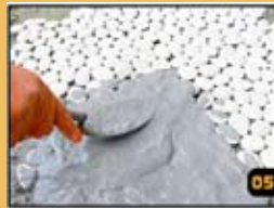
05 It is recommended that the pebbles be sealed with a quality impregnator before grouting and again after the grout has dried.
